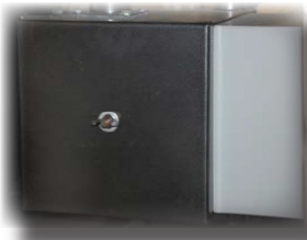
HEPA filter assembly with cover installed
